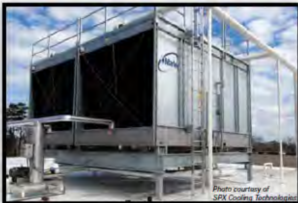
SPX Cooling Technologies utilizes Green Bull specialty services for fixed ladder cooling tower applications
